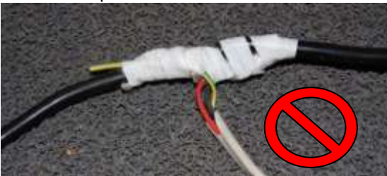
More examples of unsafe cords:
